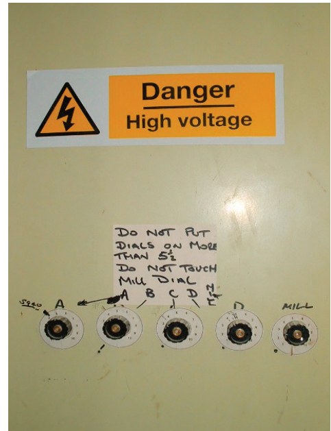
Figure 4. Shocking example of a very poorly maintained system.
