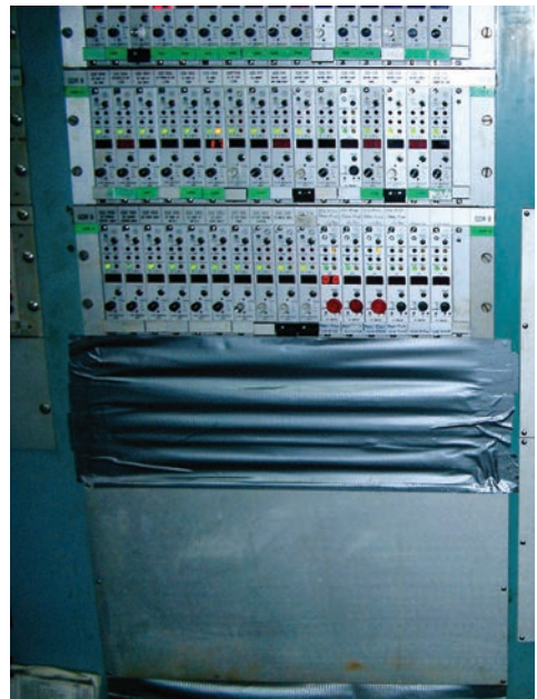
Figure 6. Using "gaffer" tape to patch a control panel is NOT indicative of a well maintained system.
