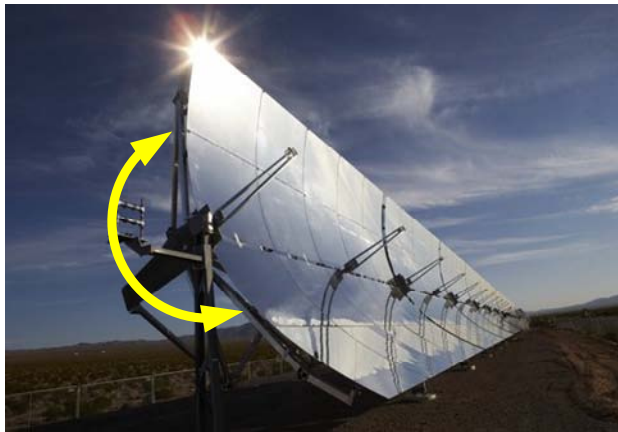
Example: Single Axis Tracker used for Solar Thermal Parabolic Trough Applications
