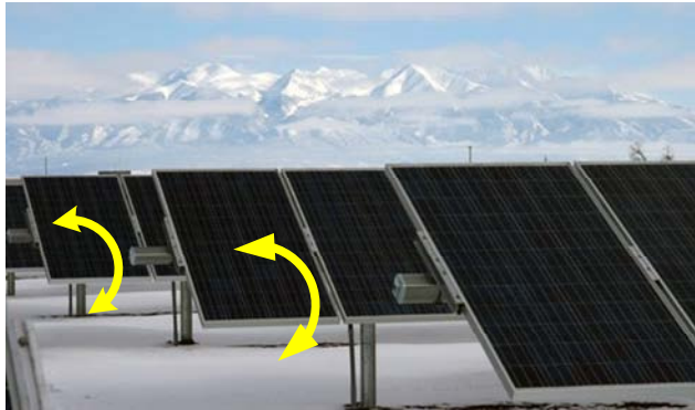
Example: Single Axis Tracker used for Solar Photovoltaic (PV) Panel Applications
