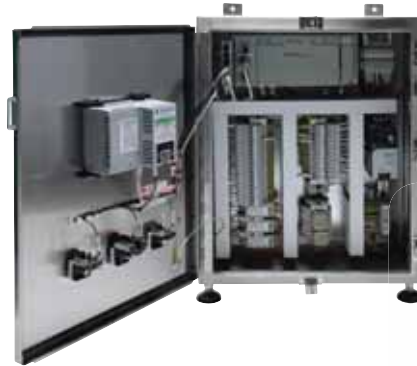
Single-Valve Steam Turbine Governor
