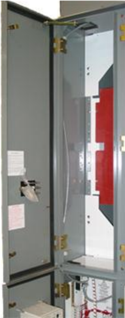
Figure 8.1 – Prepared Space with “Bypass” Cable to Lower Panel
