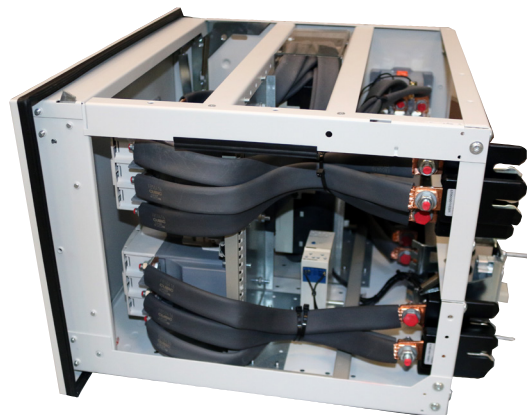
Connection: Between electrical components.
