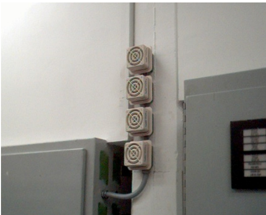
The use of single tone horns could drive up asset inventory when multiple tones need to be triggered.
