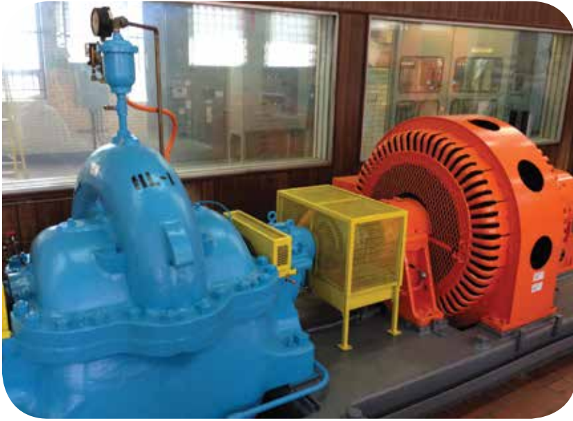
The onboard MPC solution enabled EnWin to mitigate pressure spikes from pump stops and starts.
