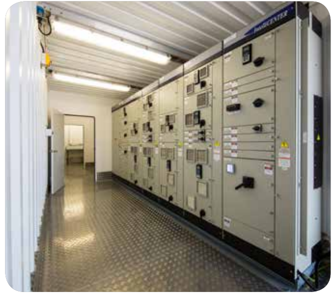
The MCC features the complete Rockwell Automation Connected Components range, including CompactLogix, E300 Electronic Overloads and PowerFlex drives all on an Ethernet backbone.
