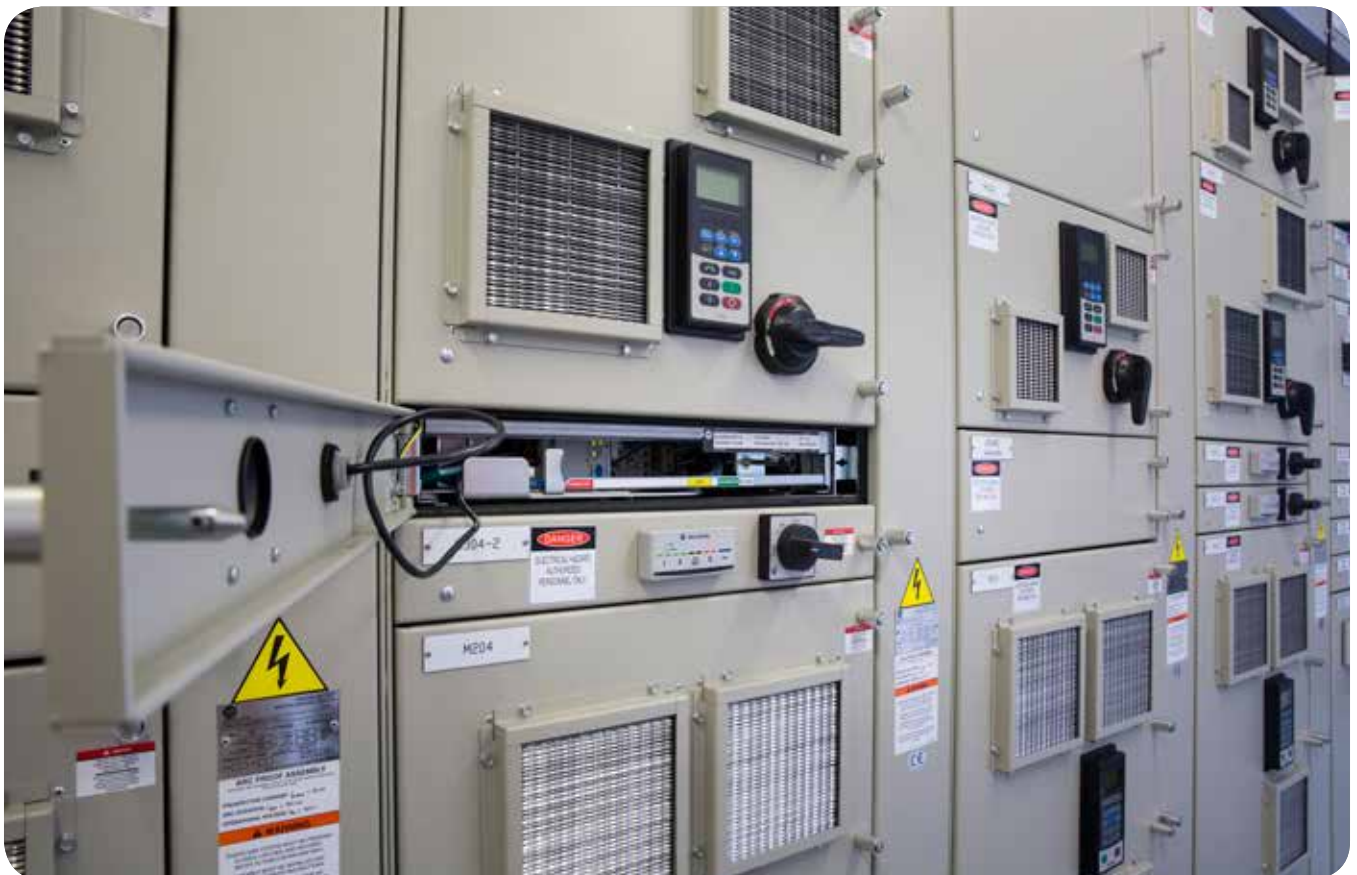
All motor control equipment has an external hardware interface module to display performance information at the front of the MCC.
