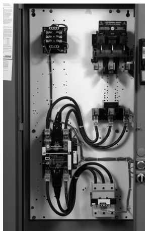
Allen-Bradley Bulletin 1232V Vacuum Pump Control Panel
