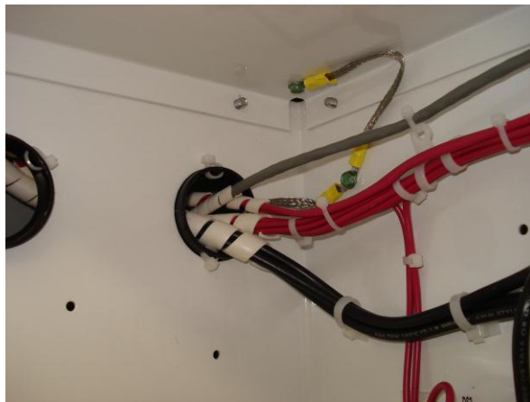
Figure 2.28 — 120 volt and XIO cables through upper cutout
