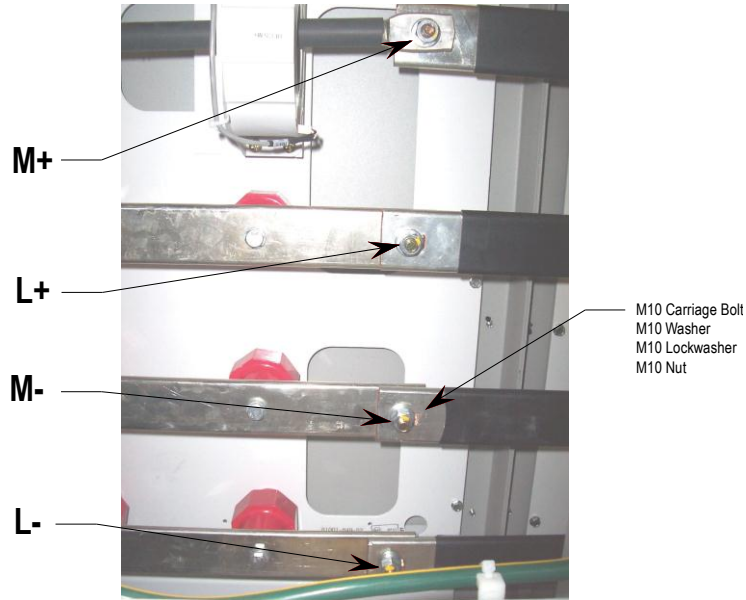
Figure 2.13 – Capacitor Cabinet (Connect left side of Medium Voltage bus pieces with M10 hardware)
