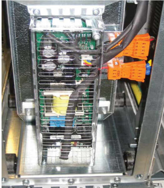
Figure 43 - LCL Filter Power Supply Assembly
