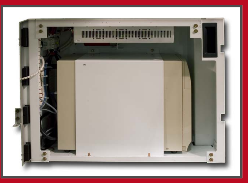
A Rockwell Automation UPS installed on a medium voltage drive in the incoming cabling section, below the LV control section keeps drive running in the event of power loss.
