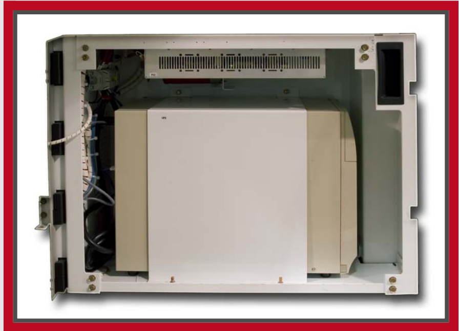
A Rockwell Automation UPS installed on a medium voltage drive in the incoming cabling section, below the LV control section keeps drive running in the event of power loss.
