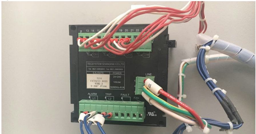
Figure 15 - Isolation Transformer Temperature Monitor (UL)
