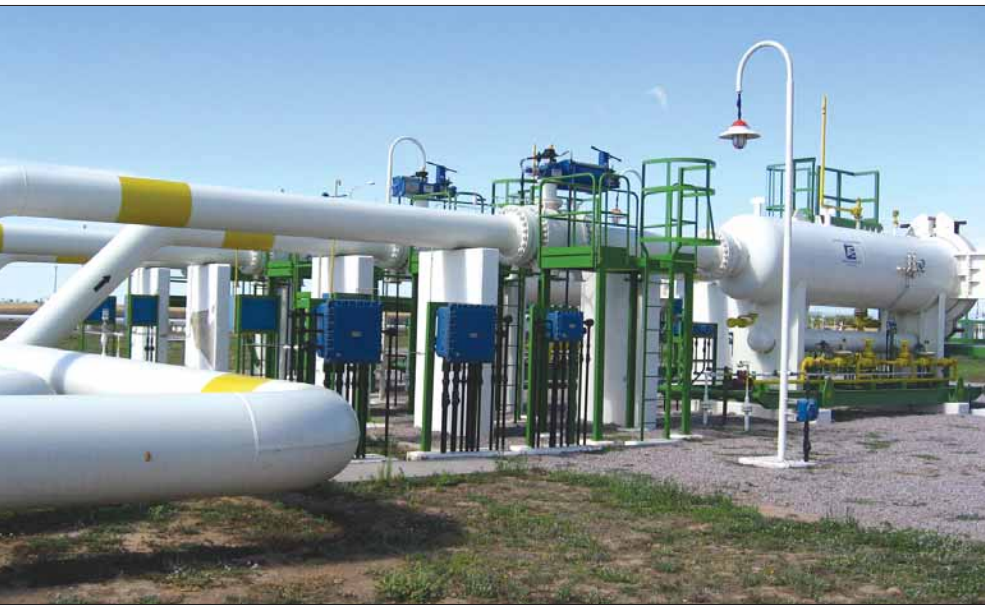
Transportadora Gas del Sur's (TGS) Bajo el Gaulicho gas compression plant is one of 16 compressor plants along TGS's 3,756-km (2,334-mile) General San Martín gas pipeline.
