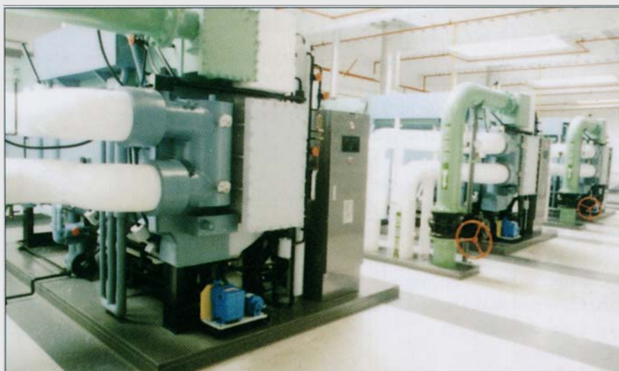
Rockwell Automation integrated control system monitors and manages three McQuay gas absorption chillers used to cool buildings, and especially the data center, at Toyota's U.S. Headquarters.
