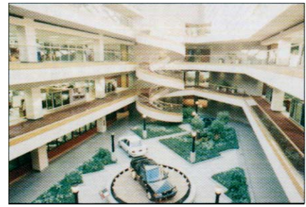
Temperatures in spaces, such as this atrium, are maintained by zoned fan/coil units connected to the chilled water system. Smart Motor Controllers manage motor functions of critical motors used to drive pumps for variable volume flow control.
