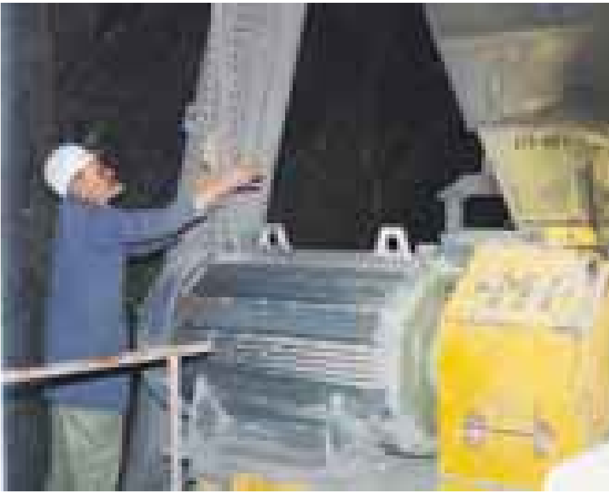
Electrical Engineer Walter Büchel on the 355 kW motor of the biggest rotary crusher that reduces 5,000 tons of stone a day. With the old time-controlled Y/delta switching system, varying charges of stone and fluctuating temperature caused problems with high starting currents. Y/delta starting in the case of the new electronic control and protection system of the 825 series is current-controlled and therefore always takes place at the right instant for minimum current.
